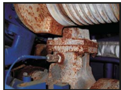
Close-up of exhaust joint
